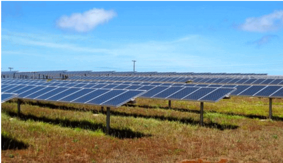
Figure I-5 LA Ola PV plant, a utility CSPV system on Lanai, Hawaii
