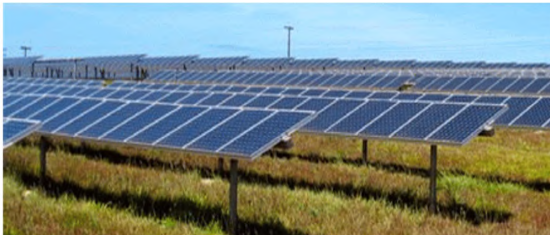
Figure I-12 La Ola PV plant, a utility CSPV system on Lanai, Hawaii
